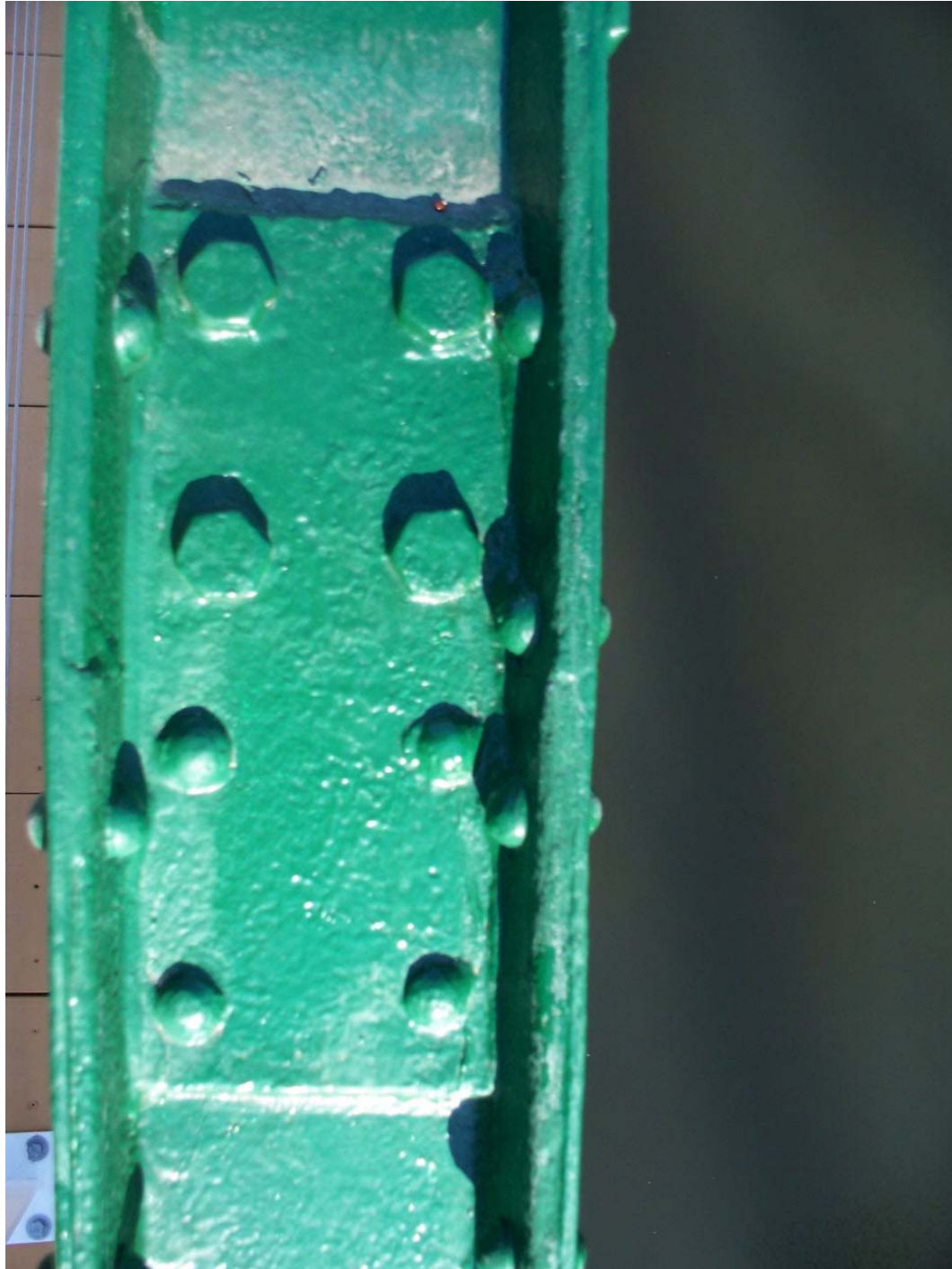
Figure 15: Detail photograph of an upper field connection for one of the channel beams following renovation. Photo by Dan Bennett, March 5, 2021.
