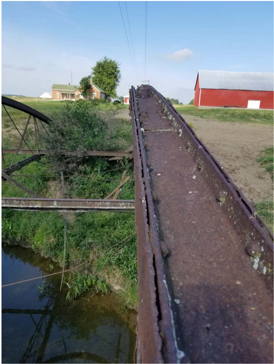
Figure 05: Condition of tube side plate, August 2020. Bach Steel Photo
