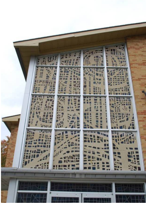
Dalle de Verre - curtain wall St. Rita's Catholic Church (1964) 5401 N. Main St., Dayton MOT-05335-09
