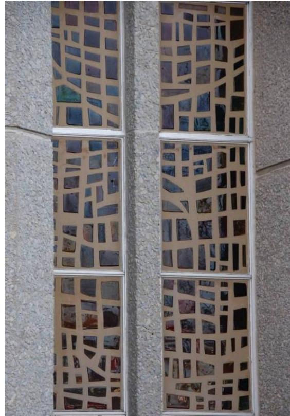
Dalle de verre - detail Church of the Incarnation (1969) 7415 Far Hills Ave., Dayton MOT-05593-03
