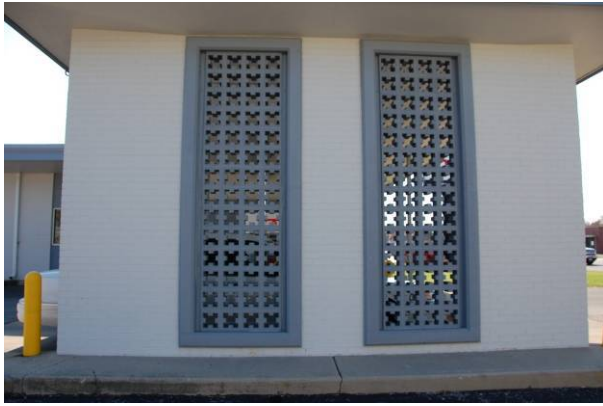
Screen integrated into façade Vandalia State Bank (1950) 4600 N. Dixie Dr., Dayton MOT-05407-09
