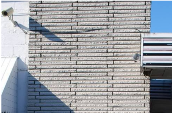
Elongated split face with offset bond Fox Cleaners & Laundromat (1947) 4333 N. Main St., Dayton MOT-05339-09
