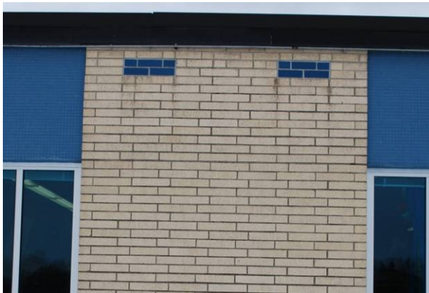
Elongated glazed brick with color accent John F. Kennedy Jr. High School (1967) 5030 Polen Dr., Kettering MOT-05496-06
