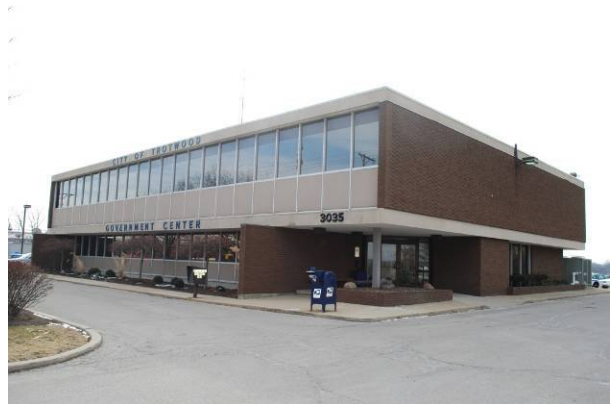
Spandrel of ribbon wall system Trotwood Government Center (1970) 3035 Olive Rd., Trotwood MOT-05469-08
