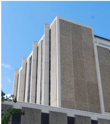
Curtain wall system Roesch Library, University of Dayton (1969) 300 College Park Ave., Dayton MOT-05158-60
