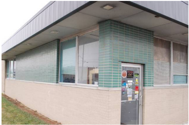
Horizontal panels of stack bond Richards Electric Supply (1961) 1569 Stanley Ave., Dayton MOT-05514-48
